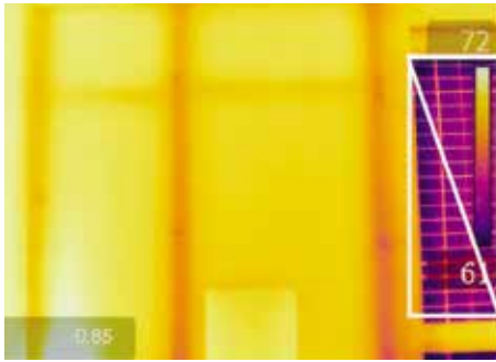
Figure 8. Interior infrared image of a wall of a college performance center and office in Philadelphia, Pennsylvania, originally built 1989.
