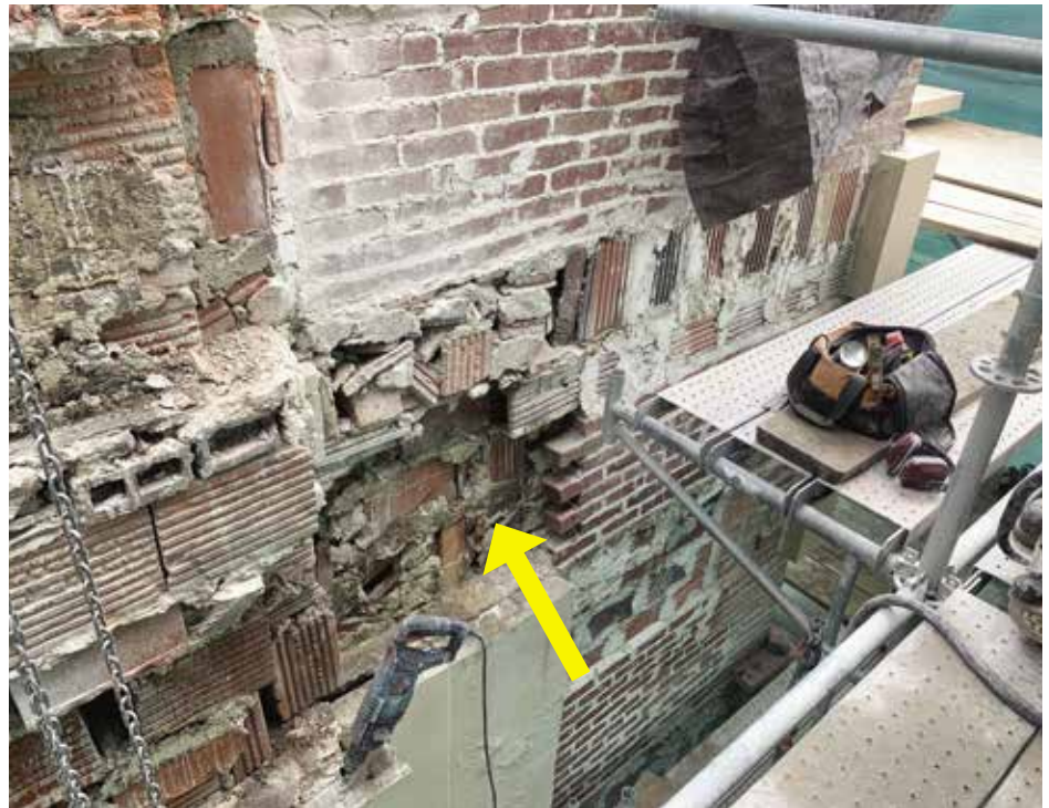
Figure 6. The removal of cast stone units from the sanctuary facade exposed structural clay tile back-up masonry. Note the void where 8-in.-deep (203-mm-deep) units were removed (arrow).
