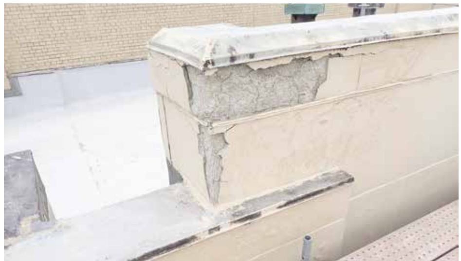
Figure 3. Cast stone units at the parapet with freeze-thaw damage and coating failure.
