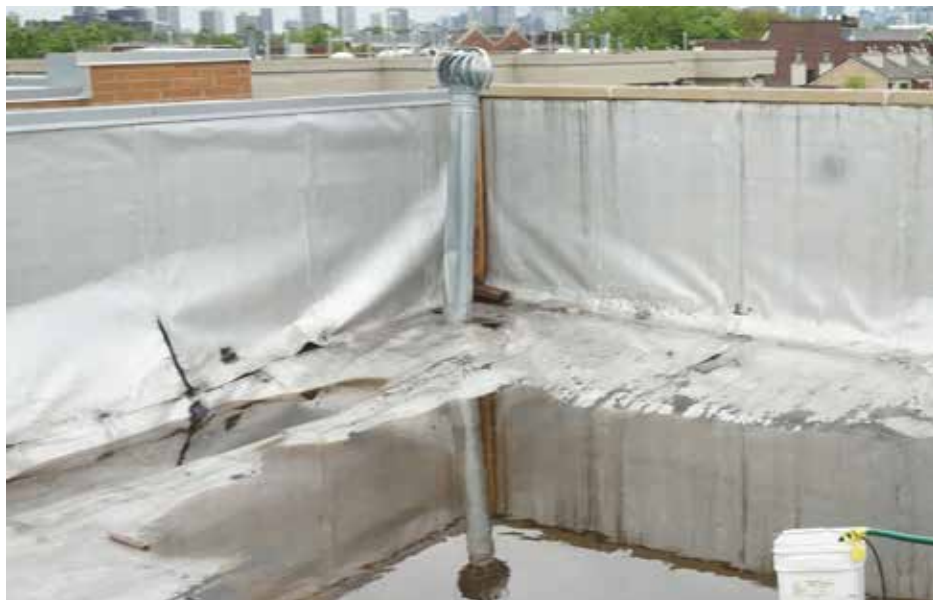
Figure 5. Turbine-style roof vent.
