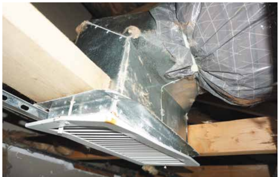
Figure 4. Zip tie connection of flexible duct to ceiling diffuser.
