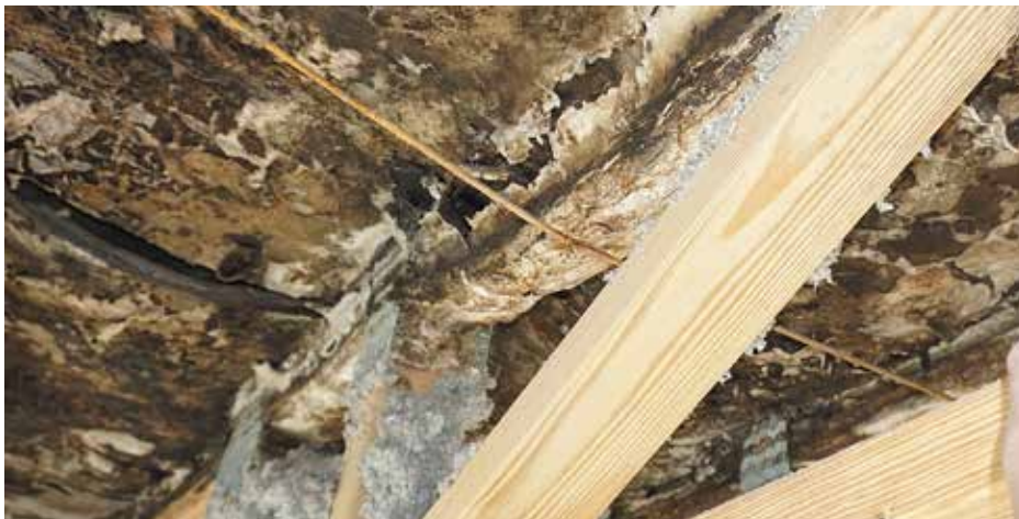
Figure 1. Sheathing and truss failure in insulated roof framing system (insulation removed to show distress).
