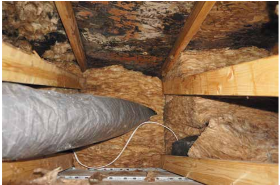
Figure 3. Ductwork within insulation.
