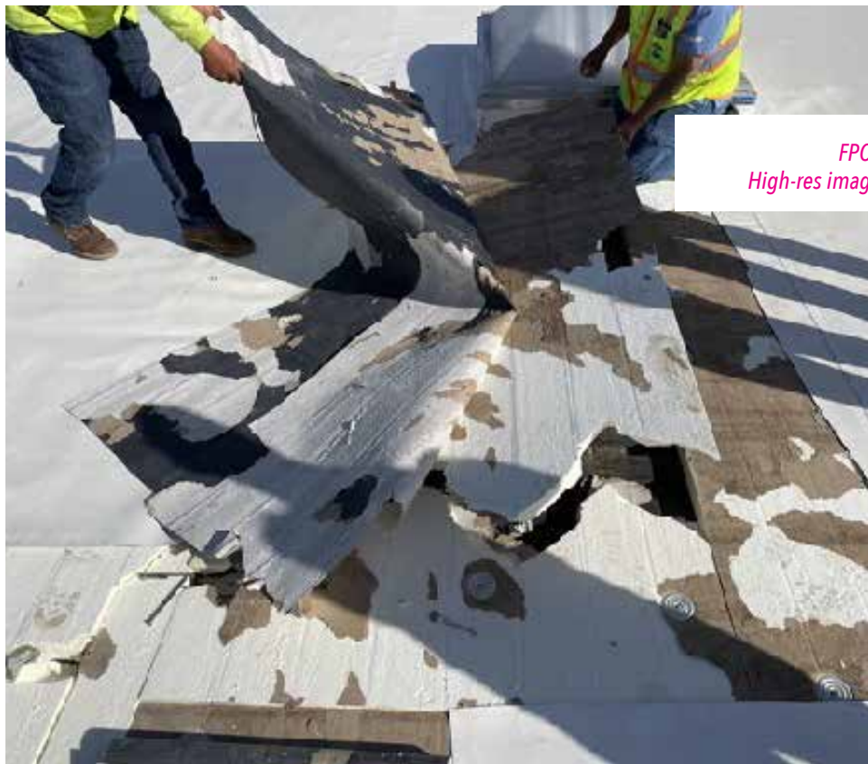
FIGURE 5. Fractured ISO with fasteners and membrane intact.
