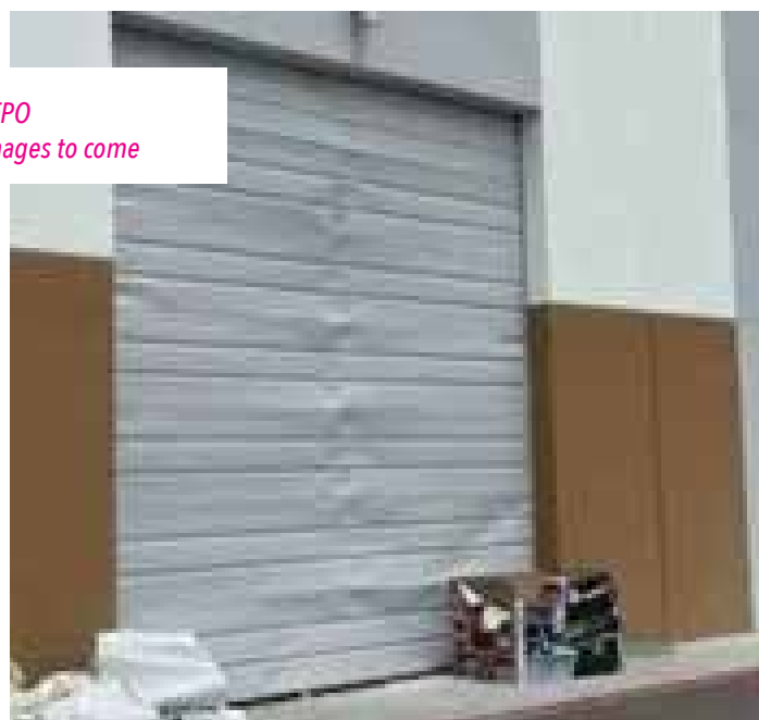
FIGURE 4. Garage door damage showing distortion from winds at or below 64 mph.
