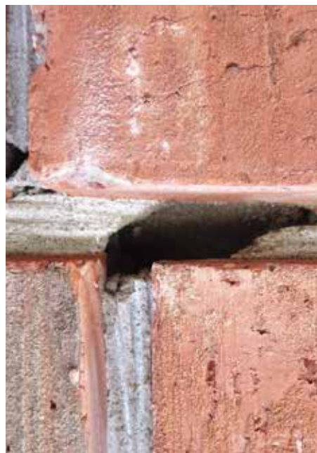
Figure 6. Voids in a mortar joint were uncovered following grinding during a repointing project.
