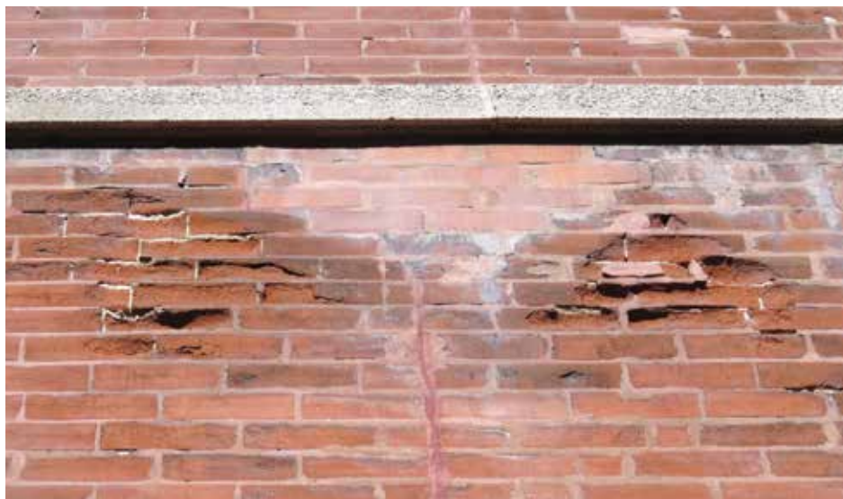
Figure 2. Various forms of exterior masonry wall deterioration.
