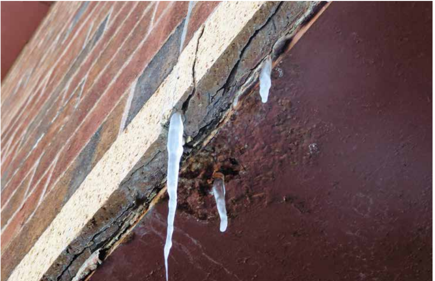
Figure 3. Deterioration of brick veneer from freezing and thawing cycles.
