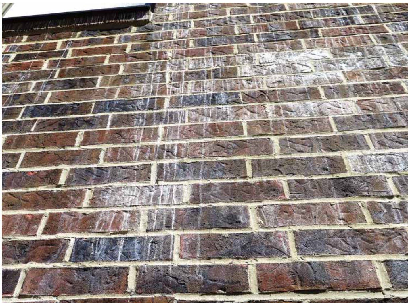
Figure 8. Water-repellent staining on an exterior masonry wall surface.
