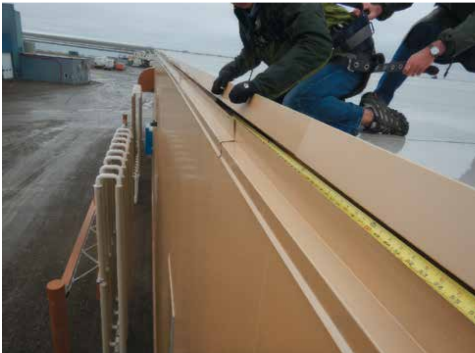
Figure 11. Failed roof edge at north elevation.
