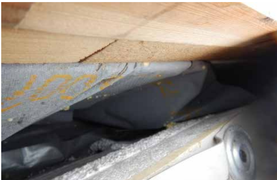
Figure 16. Membrane under tension at washer.
