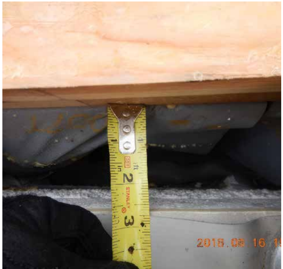
Figure 15. An approximate 2-in. gap was observed at both openings.
