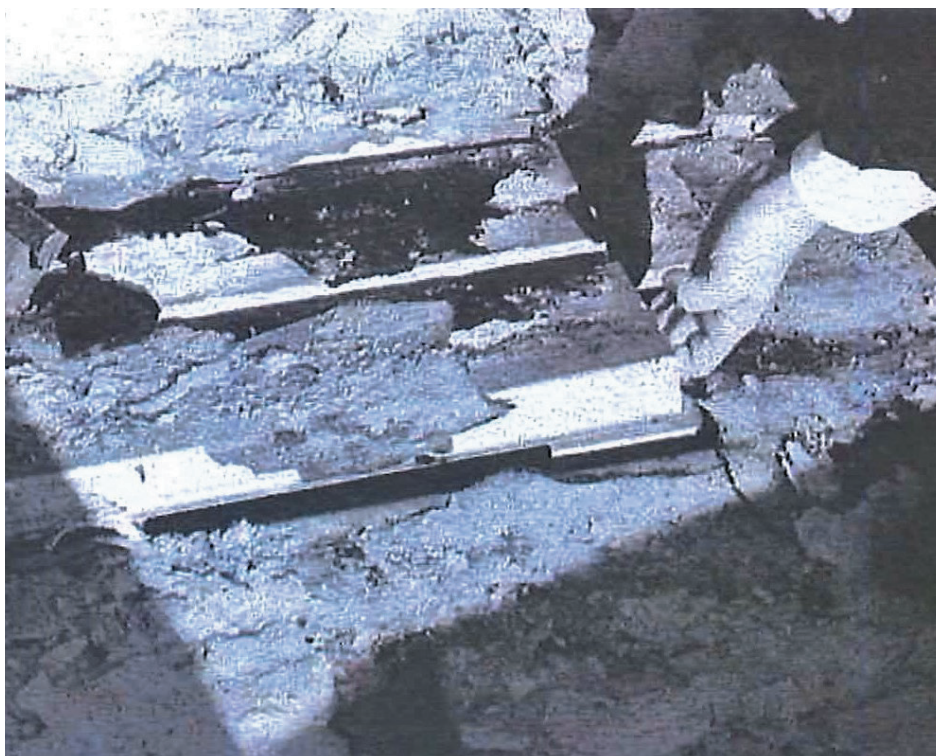
Figure 2. Loose decking revealed in the course of a tear-off project.
