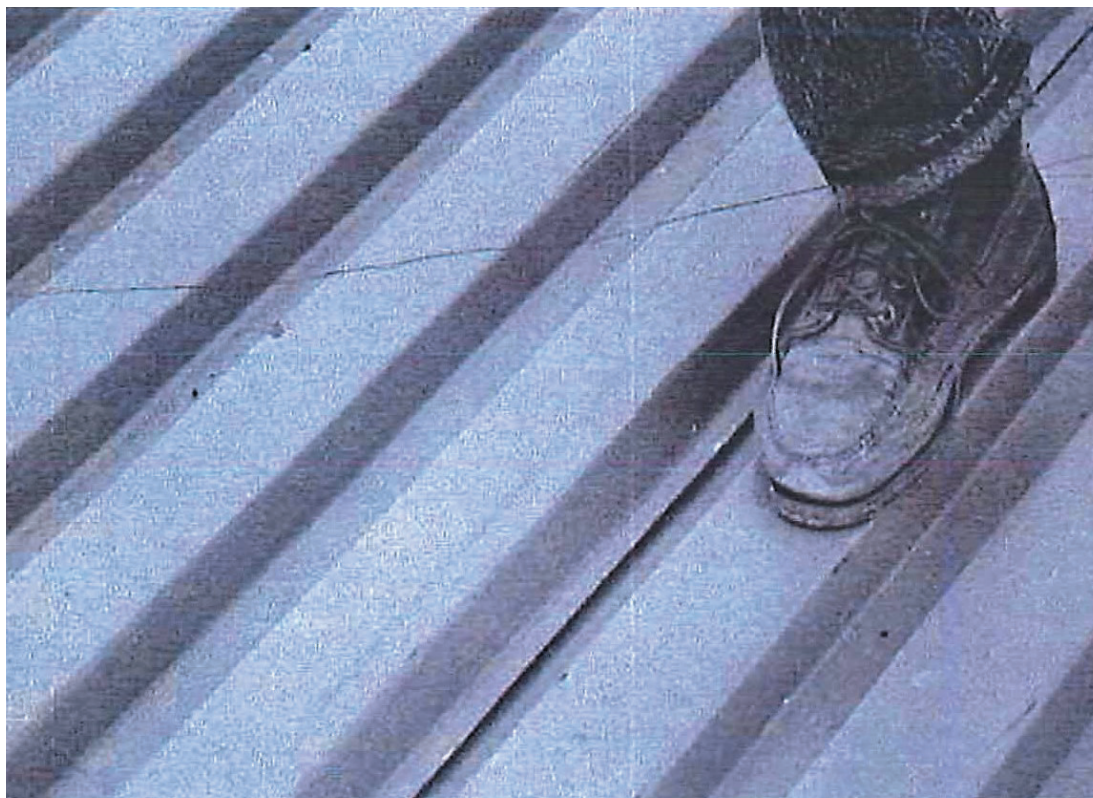
Figure 3. Inspection showed that sidelap attachment is absent here. The deck cannot perform as a shear diaphragm without sidelap stitching screws (or another connection method).
