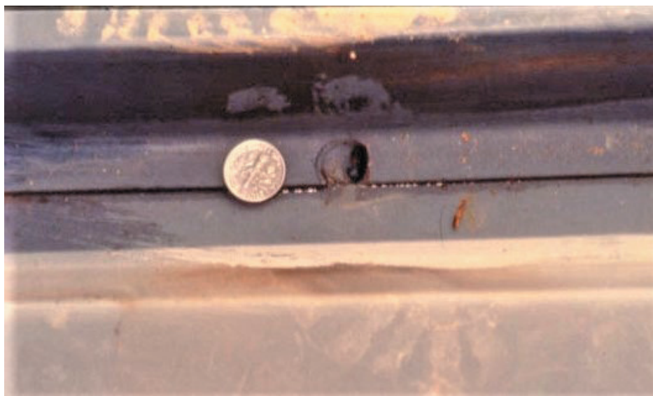
Figure 6. Work of this nature (undersized welds) can quickly reveal the skill of the welder. When \frac{3}{4} -in. (19-mm) weld is specified but the weld size is smaller than a dime (that is, less than 0.7 in. [18 mm]), corrective action for proper welding is required. This can mean going over most or all welds on a project with a second pass.
