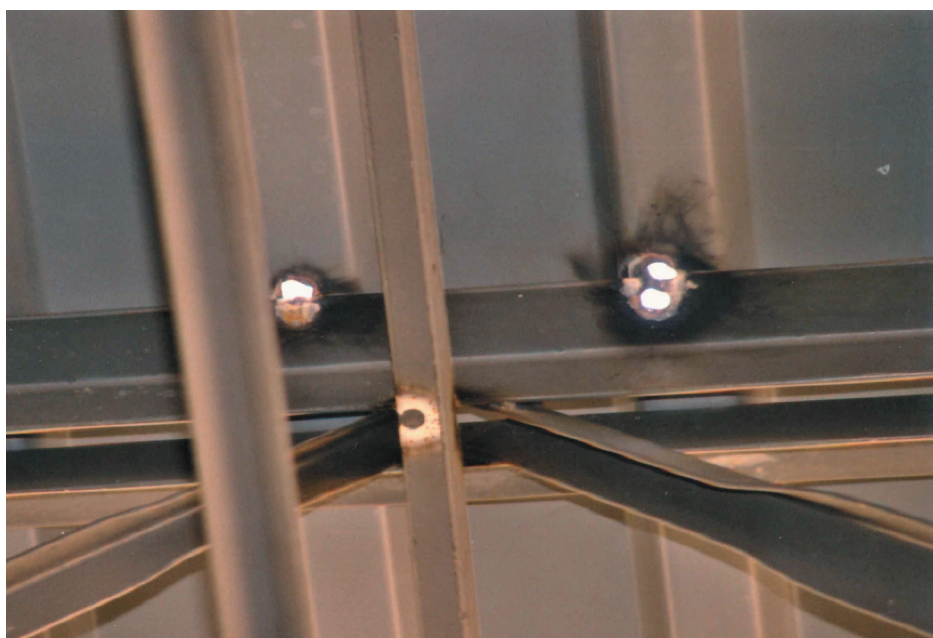
Figure 4. Complete “blow-through” of the top chord of joists is shown here. This reckless welding completely degrades the load-carrying capacity, and considerable rework will be necessary.
