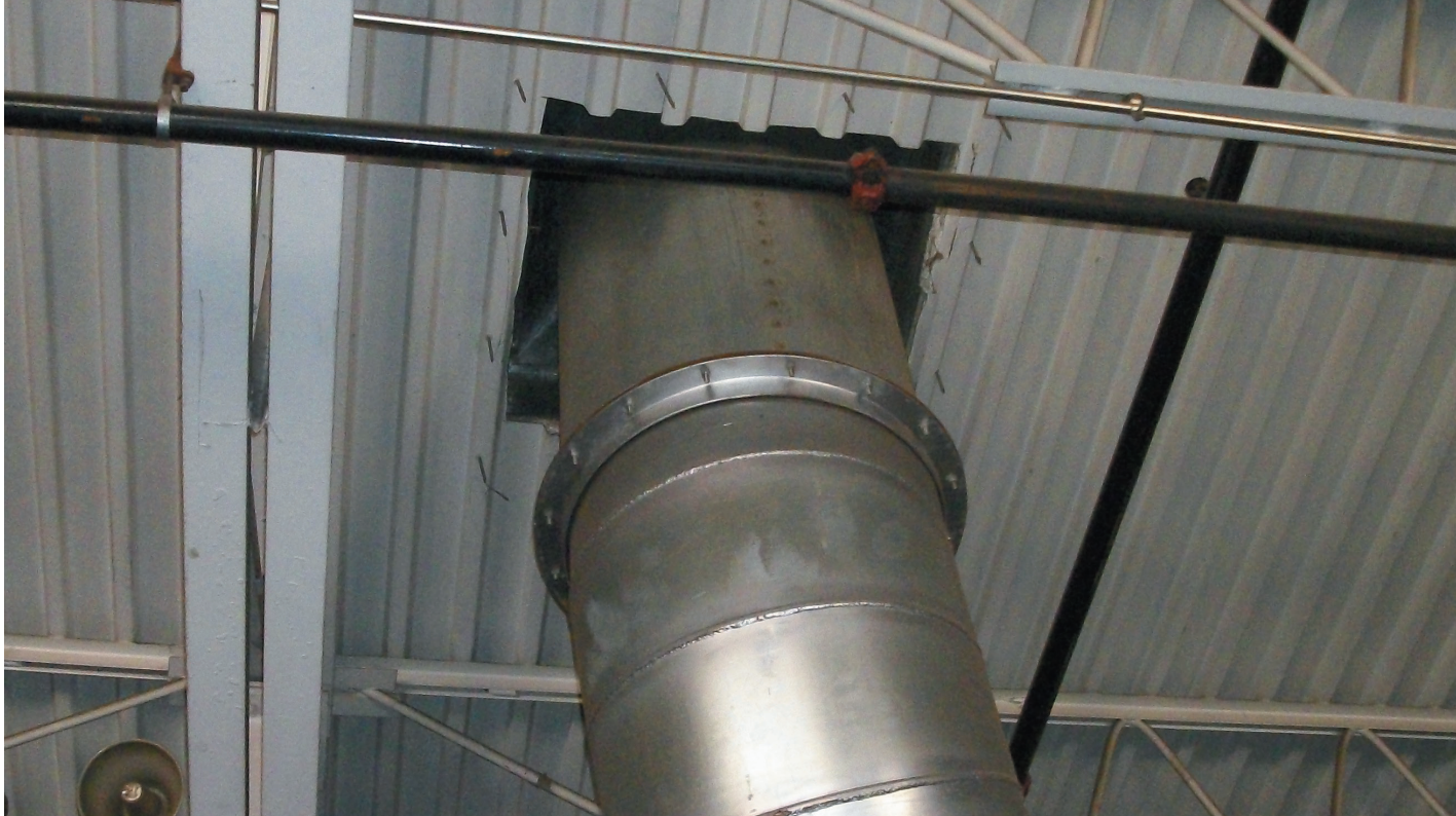
Figure 8. Unframed openings can be a serious defect, especially at large penetrations. Cutting out five ribs (as shown here) will make the deck go as soft as a couch cushion.
