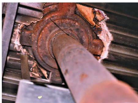
Figure 10. A below-deck clamp is needed to bring the drain components together tightly. A drain assembly is not complete until clamps are installed—both above and below. Note that four-side framing is missing at this opening.
