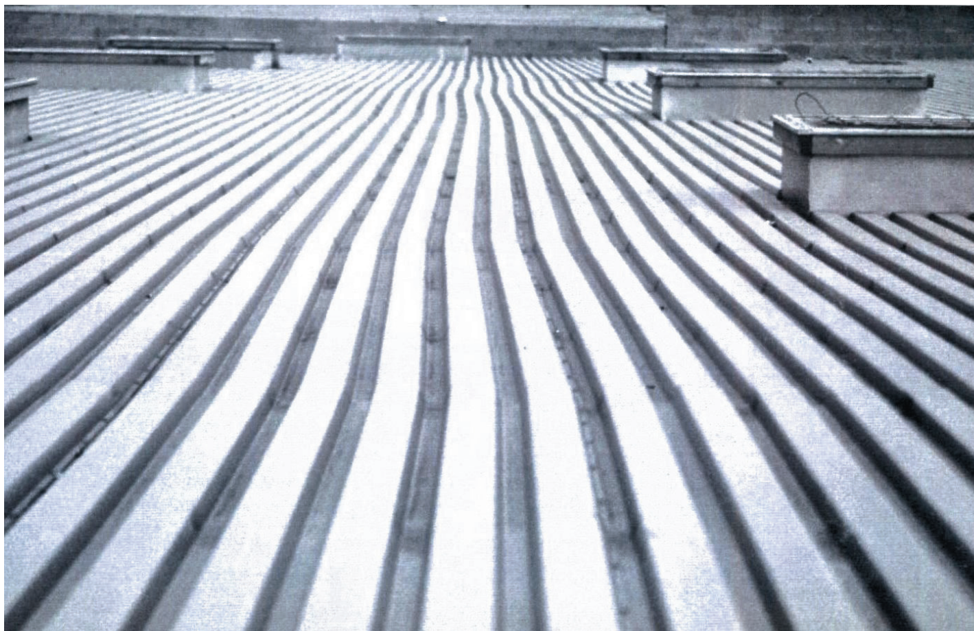
Figure 16. A meandering deck may well portend that other aspects of work are of substandard quality.
