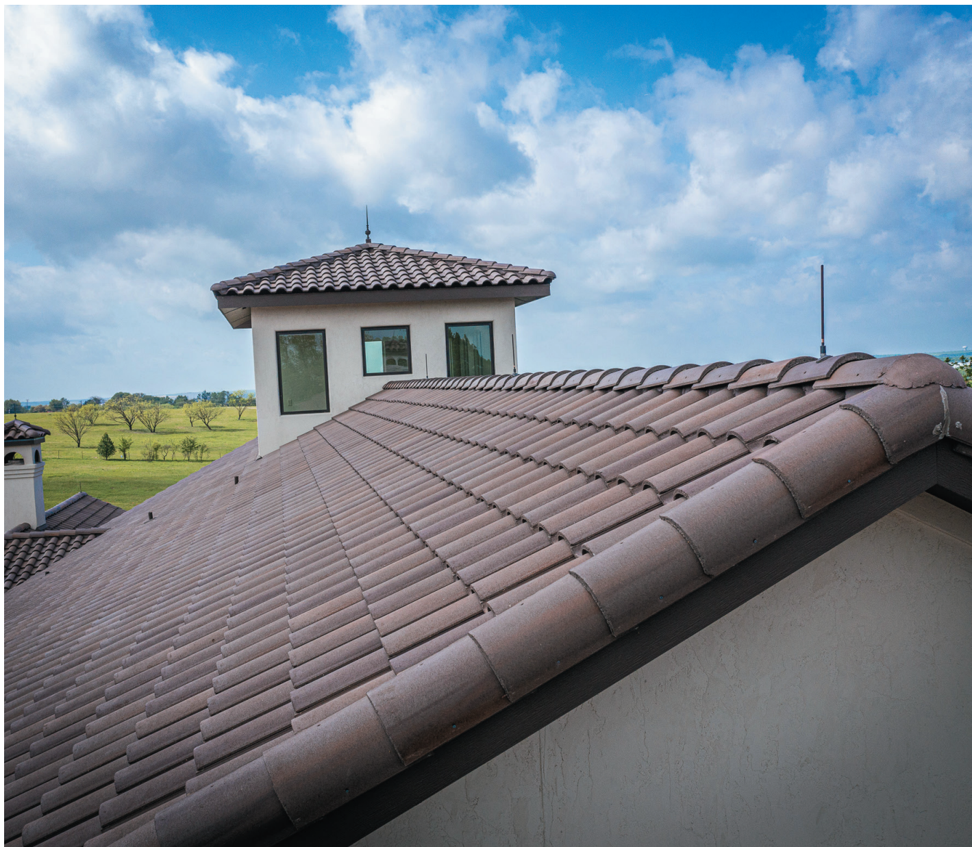
Figure 7. Texas home protected with a lightning protection system. Credit: Bonded Lightning Protection Systems, Ltd./Texas; to learn more about this project, visit lightning.org/most-innovative-design-award-2 .
