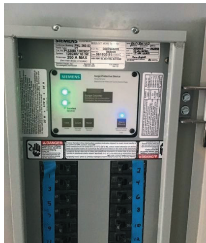
Figure 3e. Surge protective devices
